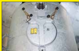
Manhole with quick opening
